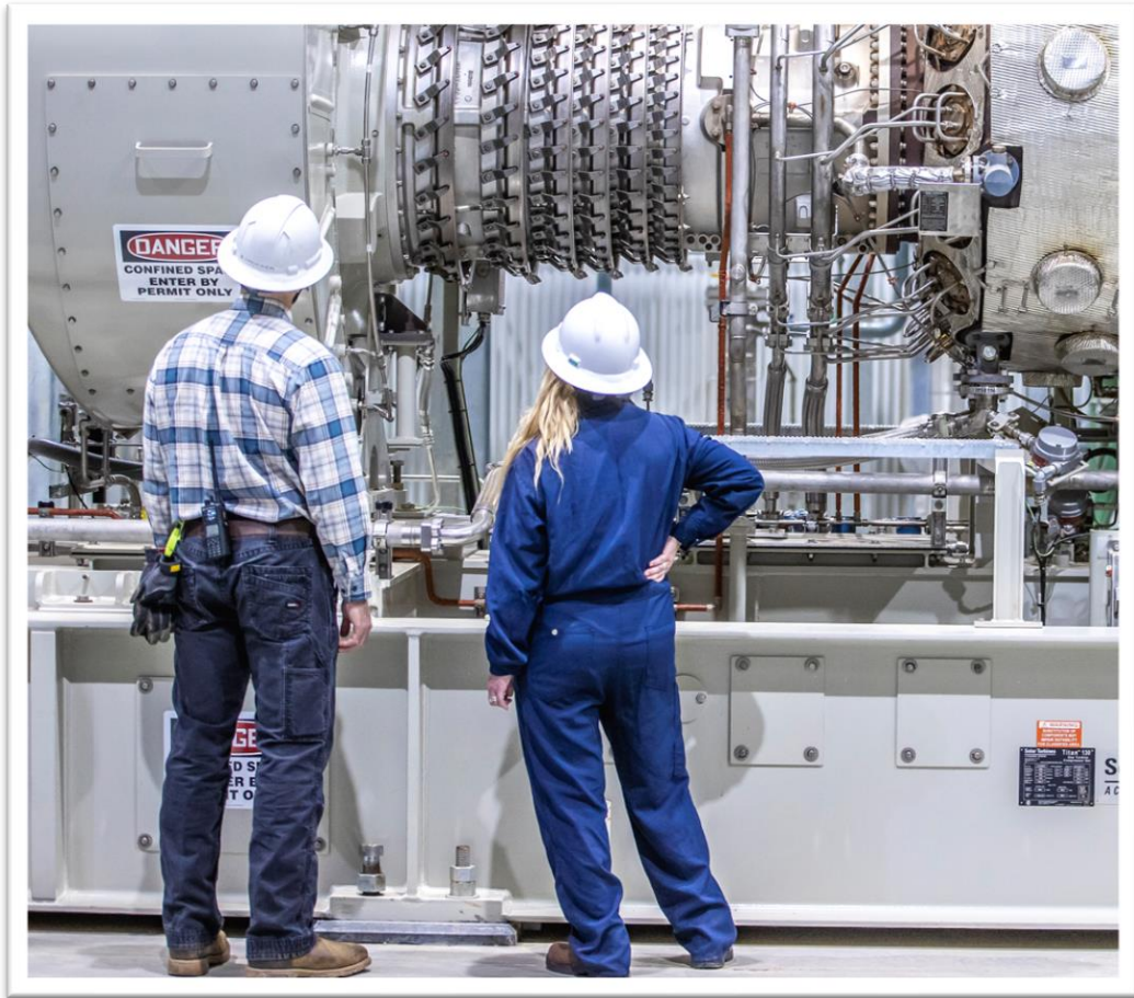
Transco Compressor Station 175 in Virginia
