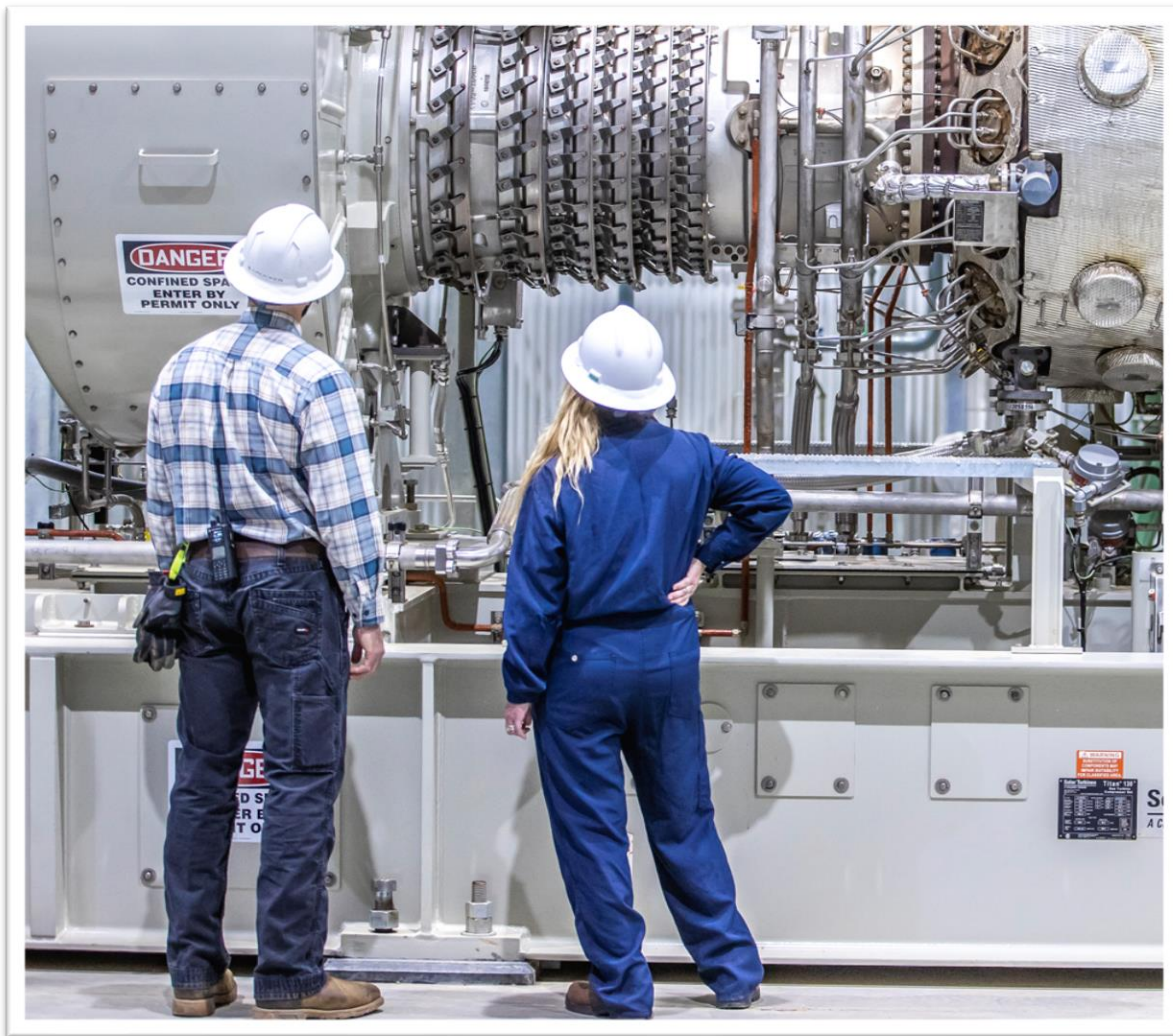
Transco Compressor Station 175 in Virginia
